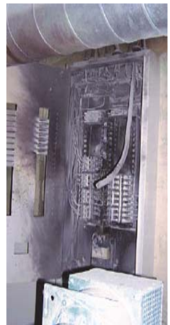
The aftermath of not turning off the power to do the job. Damage to worker and equipment is substantial.
