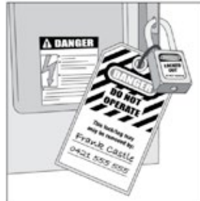
Picture 5: A personal danger tag advises who to contact about the work and warns that operating the plant could put the worker's health and safety at risk.
